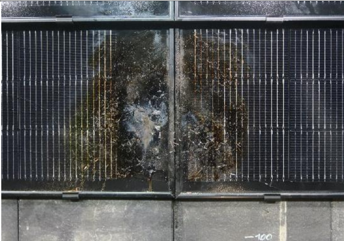
Fig. 27: Solarstone tiled roof kit, Test set-up (test 3) – Damage front side
