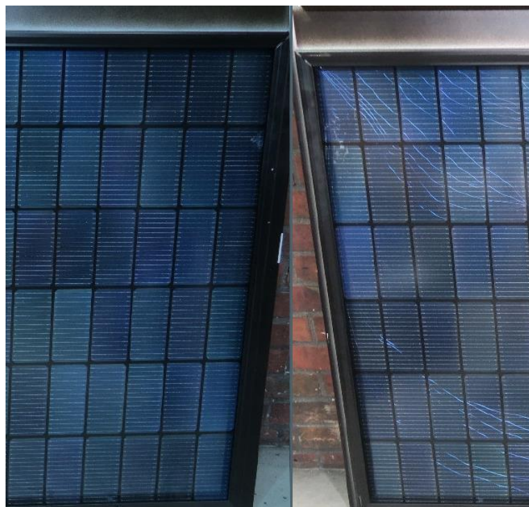
Fig. 16: Solarstone full roof kit, Test set-up (test 3) – Damage back side
