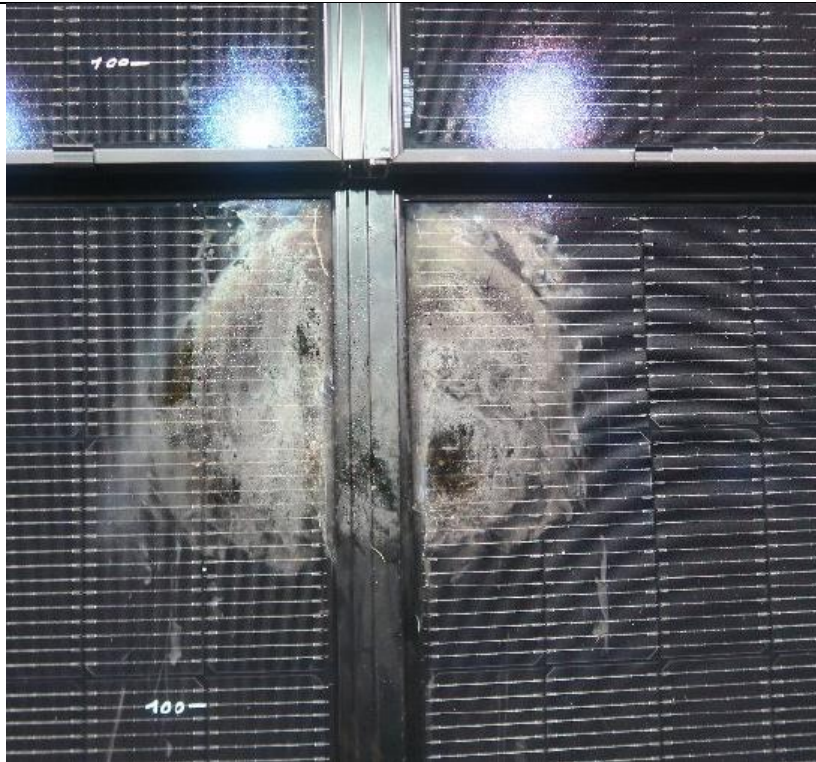
Fig. 15: Solarstone full roof kit, Test set-up (test 3) – Damage front side
