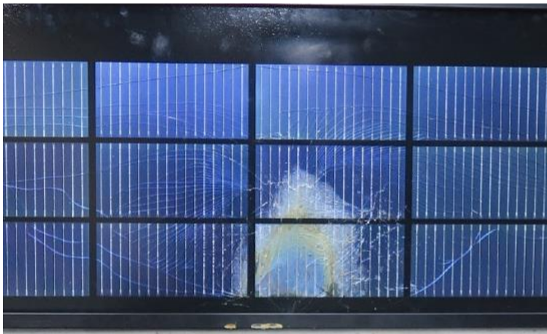
Fig. 20: Solarstone tiled roof kit, Test set-up (test 1) – Damage back side
