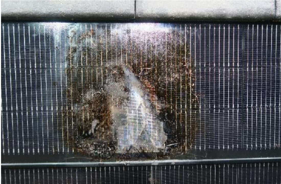
Fig. 19: Solarstone tiled roof kit, Test set-up (test 1) – Damage front side
